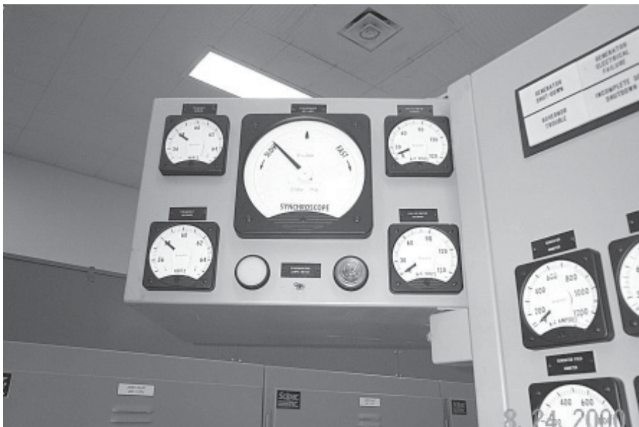
Figure 4: Photo of typical synchronizing meter panel
